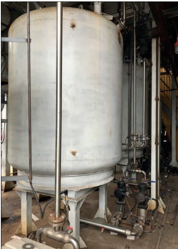
Fig. 4. Pilot-scale biogas installation of Eco-Energia LLC with a reactor volume of 2 m 3
